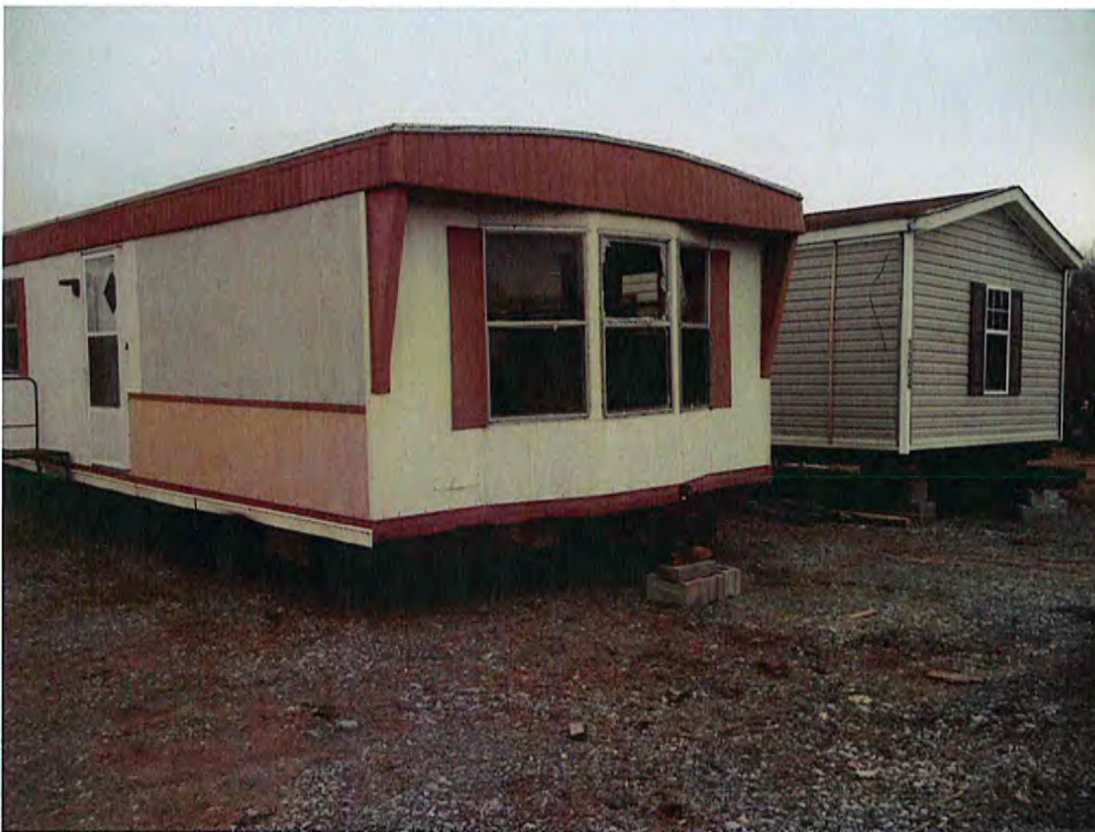
Date: 01/31/2014 Time: 2:42 p.m. Direction: NE Photo by: M. Stevenson Exposure #: 002 Comments: waste mobile home, broken window.
