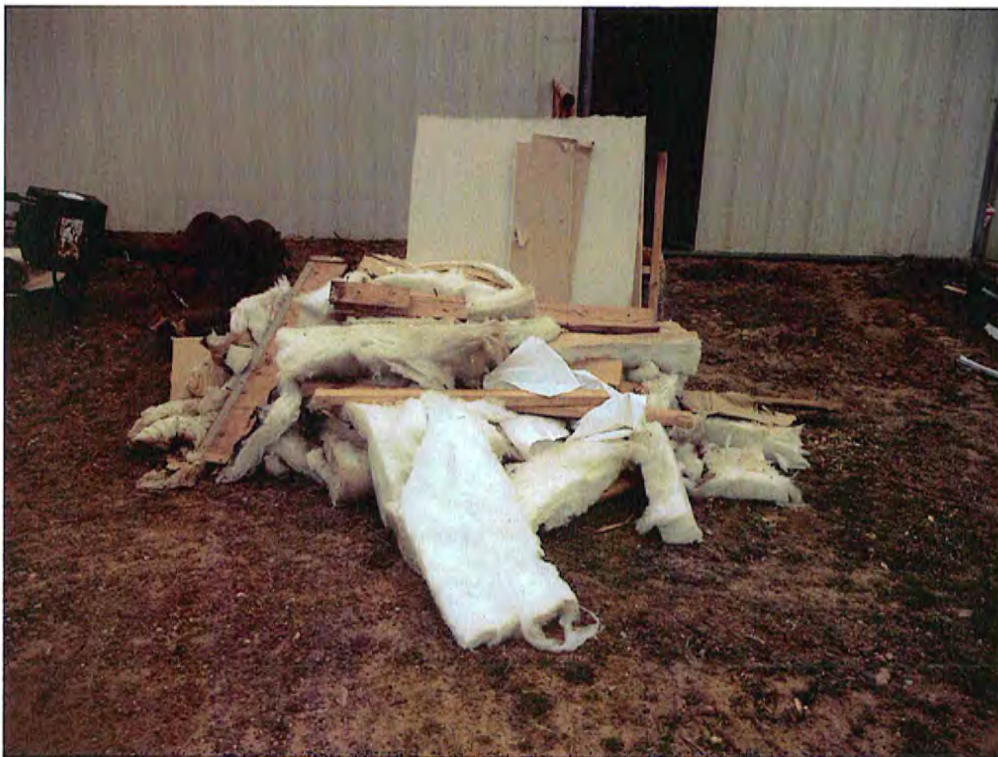
Date: 01/31/2014 Time: 2:49 p.m. Direction: N Photo by: M. Stevenson Exposure #: 010 Comments: insulation, dimensional lumber, drywall, misc.
